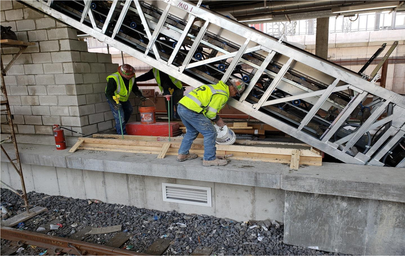
ST Platform Plumbing Closet Room
