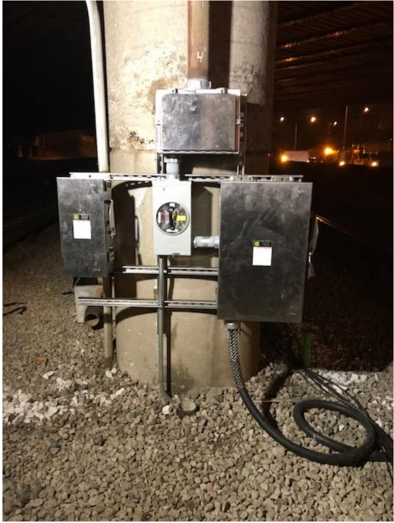
Foster Relay House Temporary AC Feed
