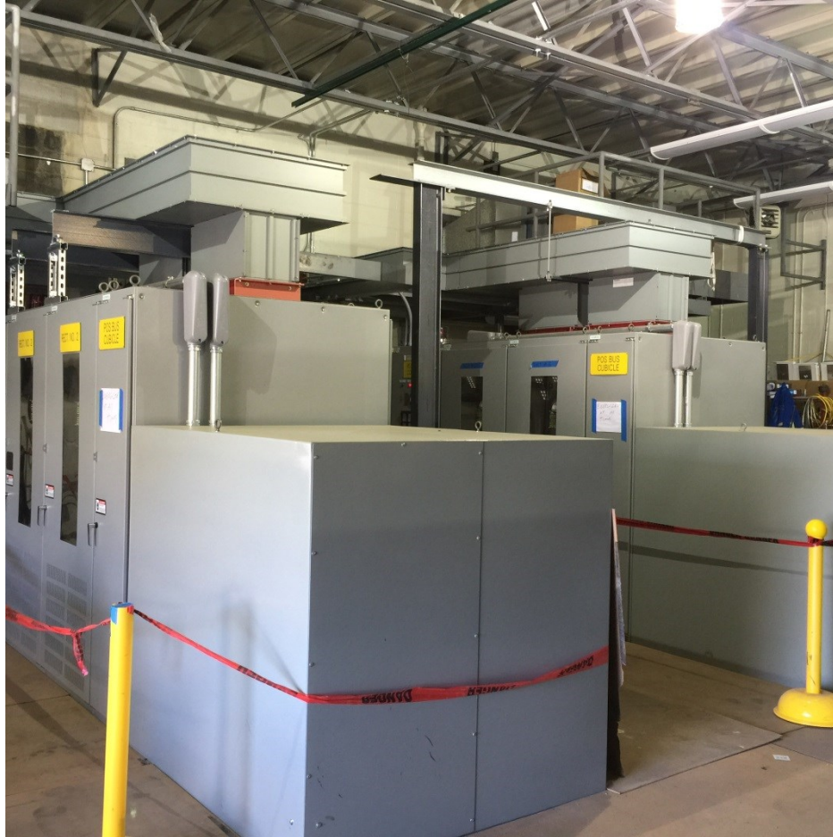
Princeton Substation: Rectifier Lineup One and Two
